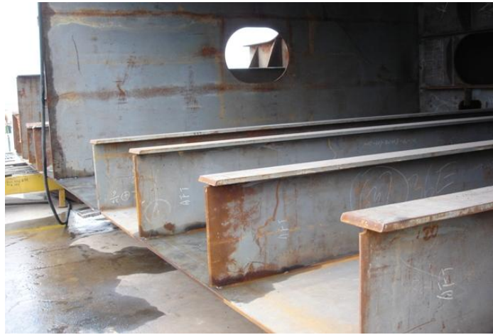
Figure 8 Shop primer damages from corrosion, welding, and mechanical at block stage
